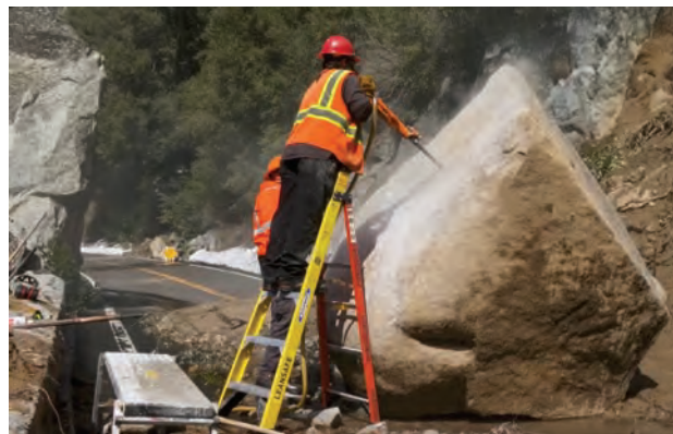
Yosemite roads and trails crew work to clear one of the many rockslides on Big Oak Flat Road with drilling, blasting and heavy equipment.
