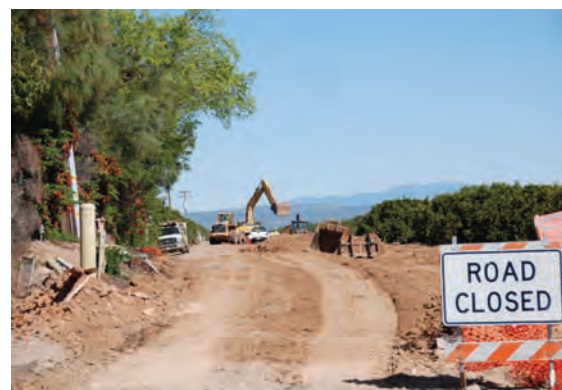
Construction on the groundwater recharge project is in full swing on the north side of Avenue 12 just west of Highway 41. (Photo Karen Petryna)
