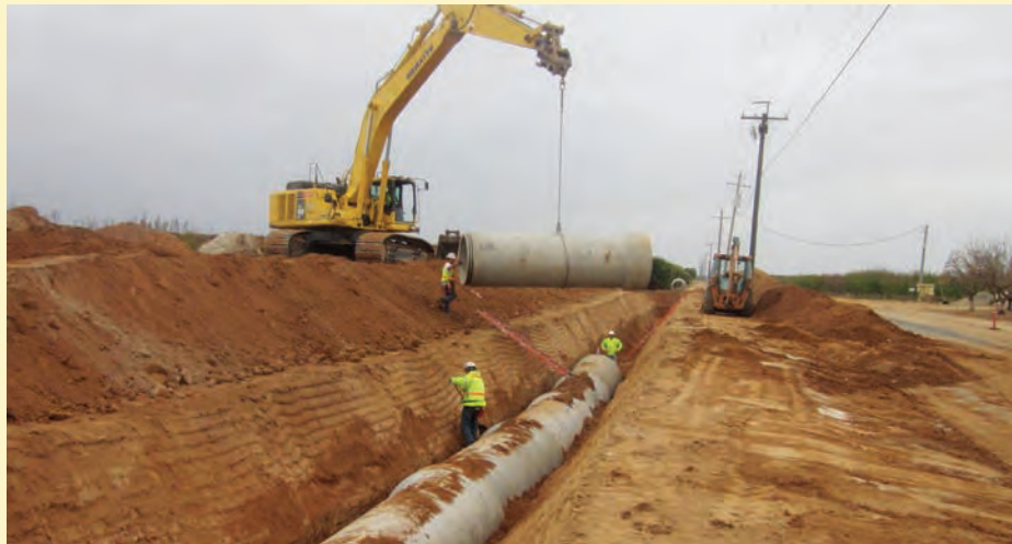
The Town Hall meeting addressed many topics, including recent activity with the Root Creek Water District, shown here installing a new 48-inch water pipeline near the new Riverstone development at Highway 41 and Avenue 12.
