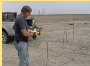
With the holes drilled, Shaw connects the antennas that will feed the information back to the computer.
