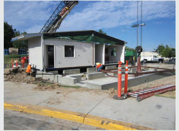
The building fits perfectly on top of its foundation to become the newest permanent building on the Sierra View campus.
