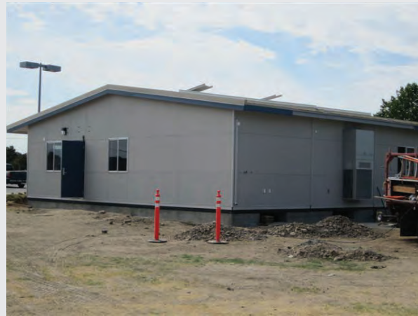
With the installation of the building on its foundation complete, interior construction is next.
