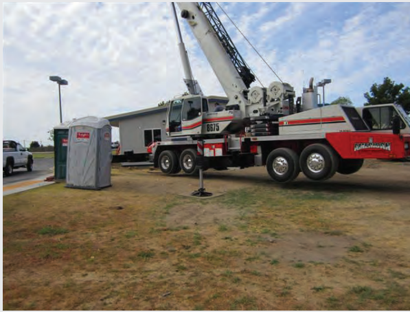
The crane gets ready to lift the new administration building into place at Sierra View Elementary.
