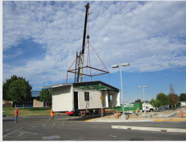
Workers guide the new modular building toward its foundation on the site where the old portable office sat.
