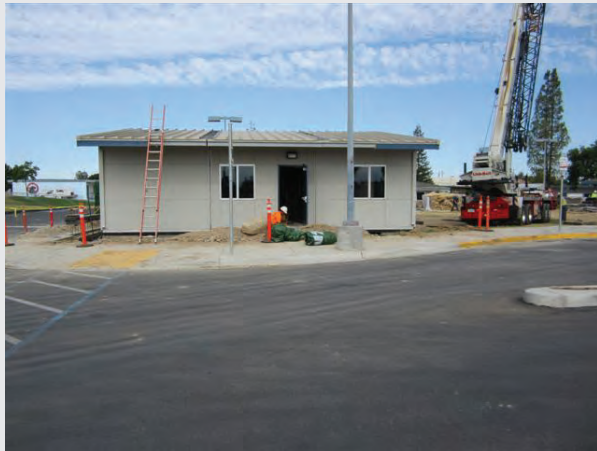
Once in place, workers complete the process of making all necessary connections for electrical and plumbing.
