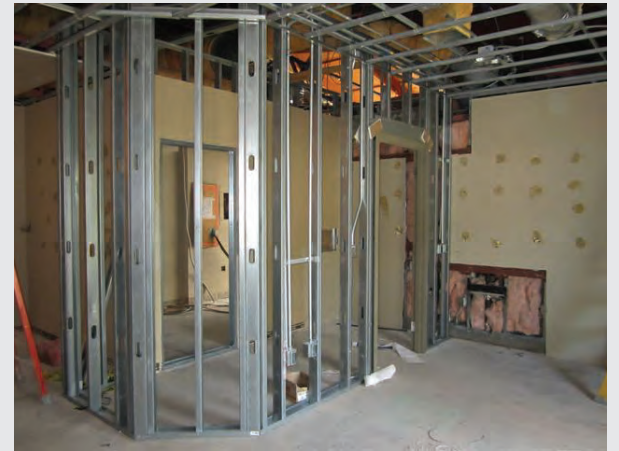
Like any other construction, walls are laid out and assembled to define the new office's work areas.
