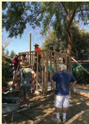
Spring Shed Construction in the capable hands of (from left) Ron Lipinski, Jan Williams, Mike Fursman and Bob Campbell.
