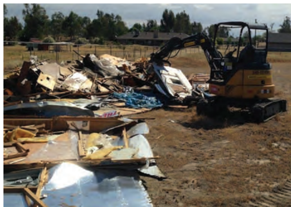
All that remains of a mobile home after a Ranchos man took a stolen excavator to the vacant property.
