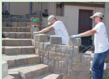
R. Lacy performs the unthinkable for concrete contractors: building up with no mortar.
