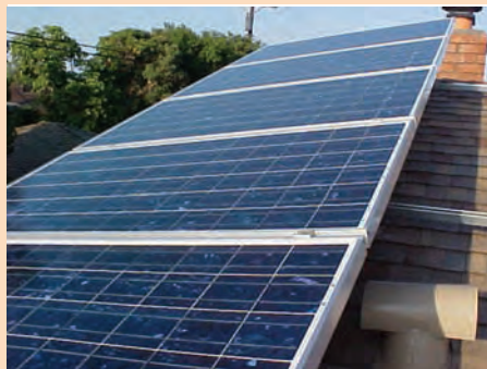
Photovoltaic panels like these will be sprouting up soon on the classrooms of Golden Valley schools.
