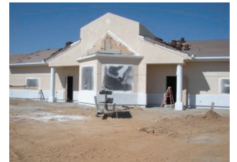
The new state-of-the-art Science Wing is scheduled for completion by October, 2010 and has been worked on continuously for the past 10 months.
