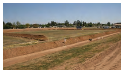
Looking southeast, the berm is gone to make way for new lights for next year's football season.
